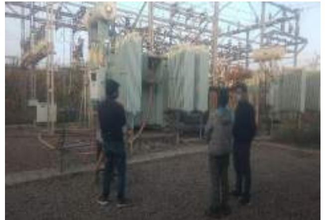
33/11 kV Khuman Lampak Sub-station
