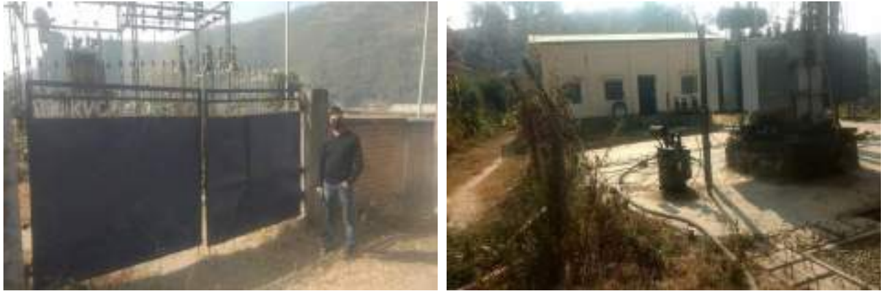
Existing 33/11 kV Substation at Litan (Augmentation)
