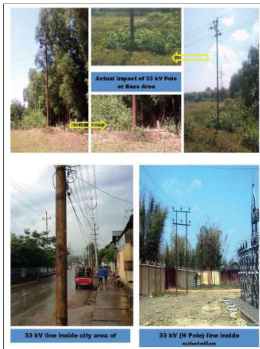
Figure 5.1: 33 kV Lines (Single & H Pole) Depicting Base Area Impact
